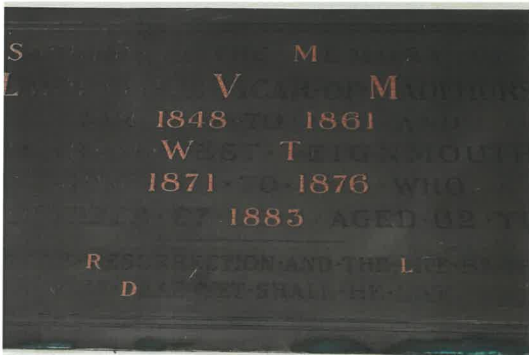
92 Monument where Lettering needs Repainting
