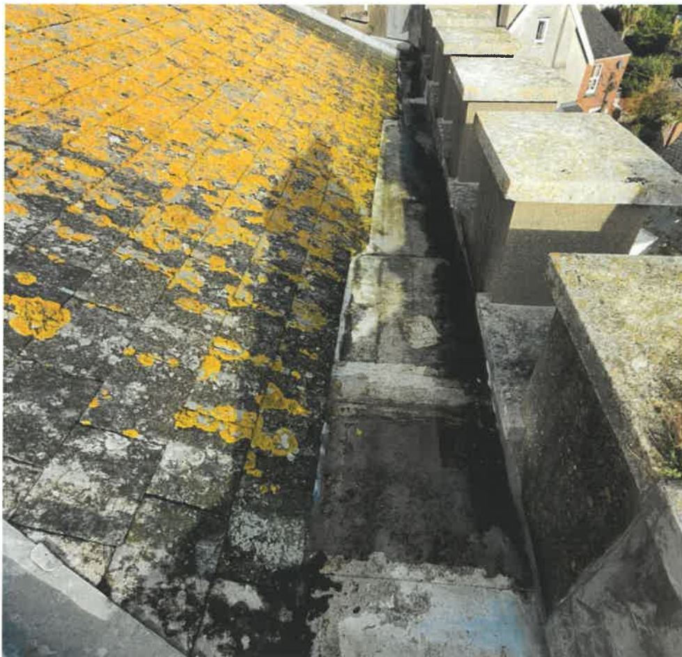
06 Overlong Valley Gutter with Flashband Repairs
