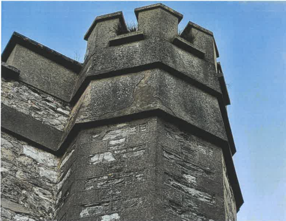
20 Render Failing to Corner Turret
