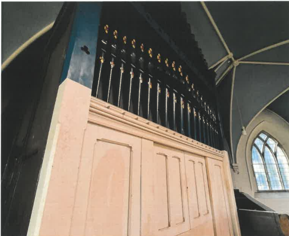
90 Organ Casing and Pipes
