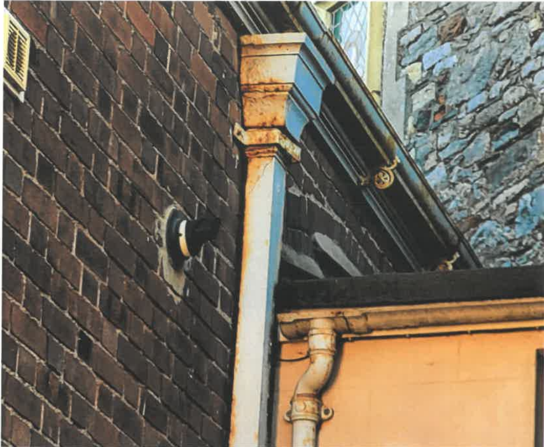
15 Rainwater Goods in need of Derusting and Decoration
