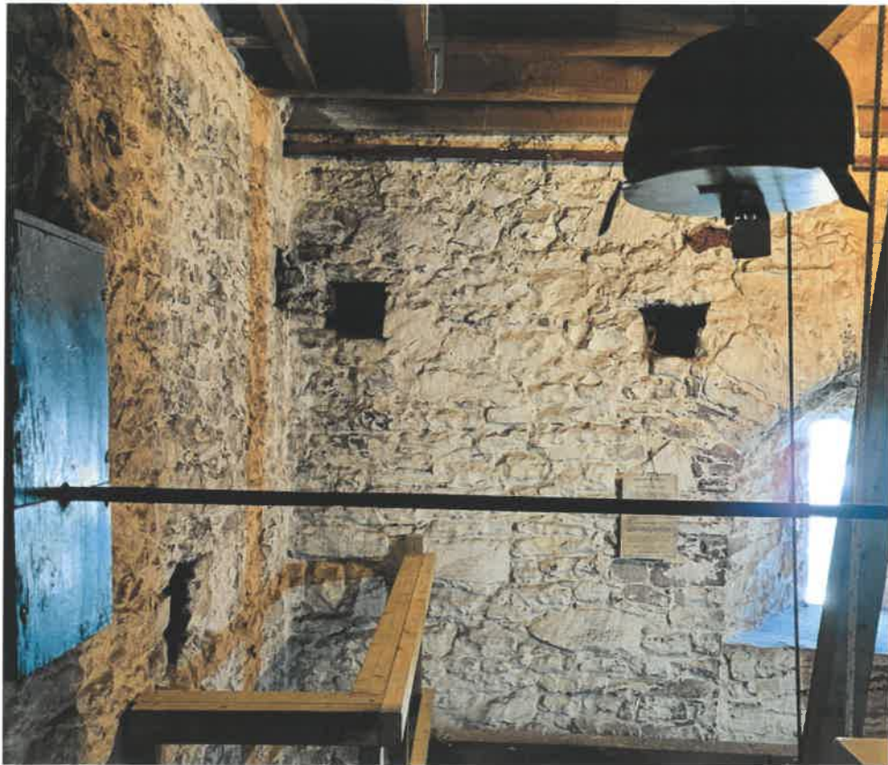
58 Sound Deadening Chamber
