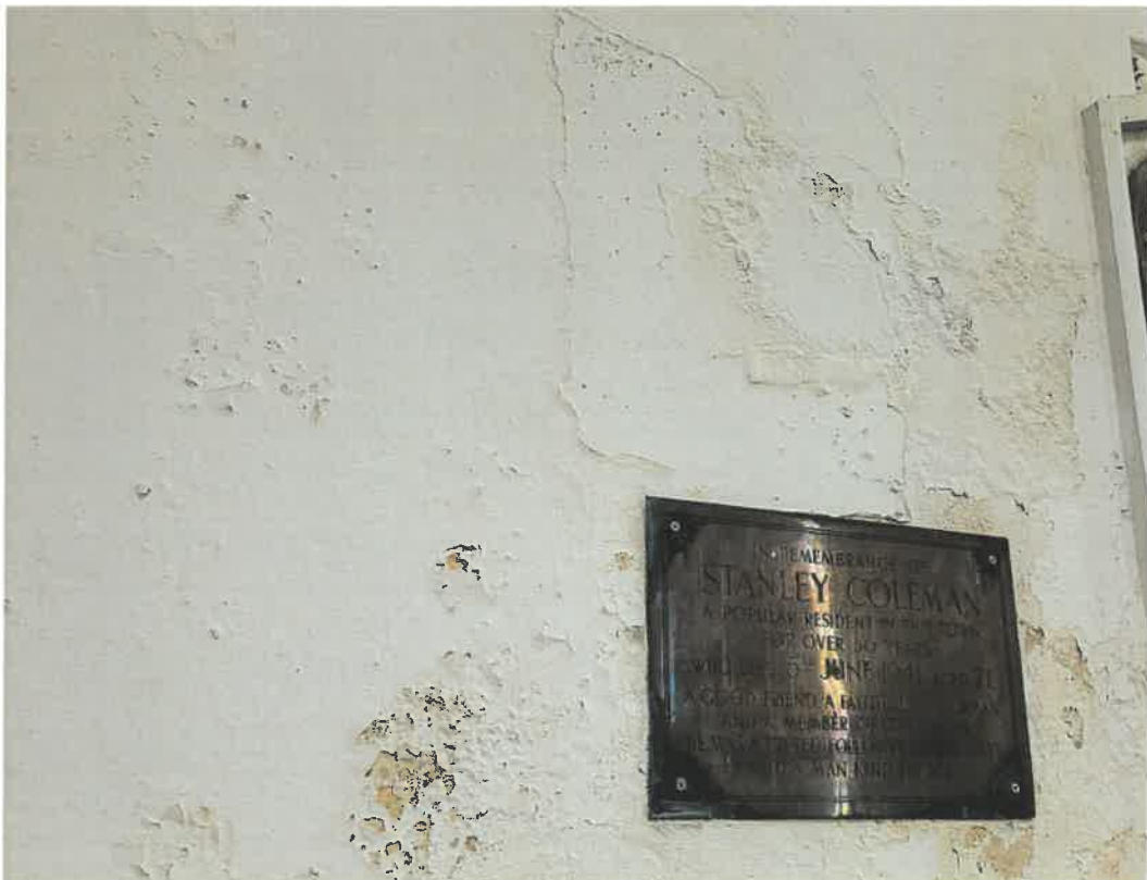
76 Damp Patch on Wall
