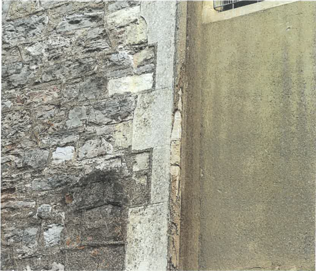
21 Render Failing to Window Quoin
